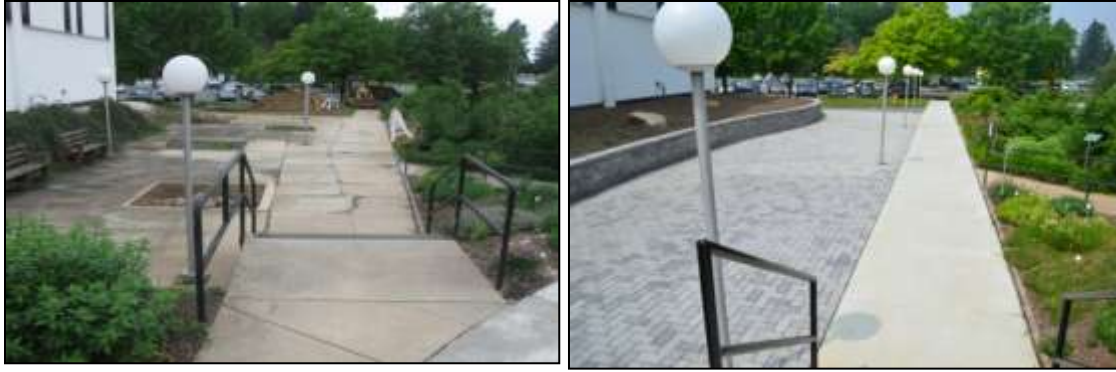
Before and after photos of porous paver installation. Photos courtesy of BCCD.
