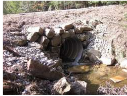
Natural stone headwalls and endwalls are built to support the roadway at pipes to prevent erosion around pipe installations.
