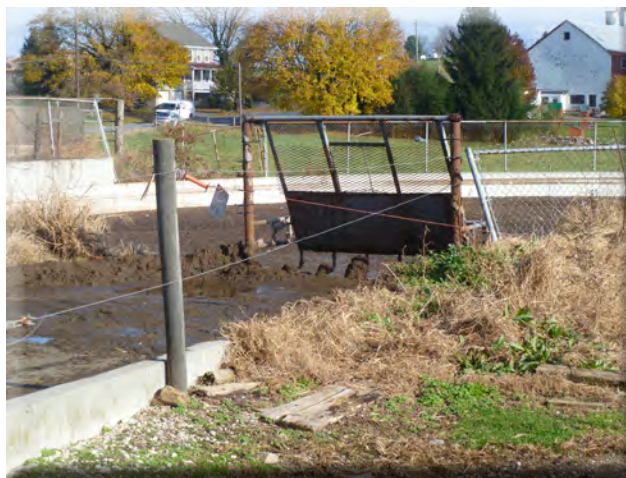
This manure storage has several safety issues, such as a gap in fence, gate left open, and signage that is ready to fall off.
